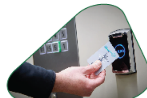
Card access at the lift
