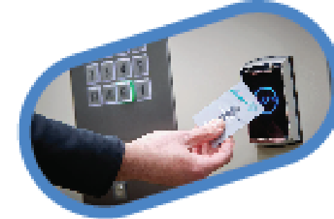
Card access at the lift
